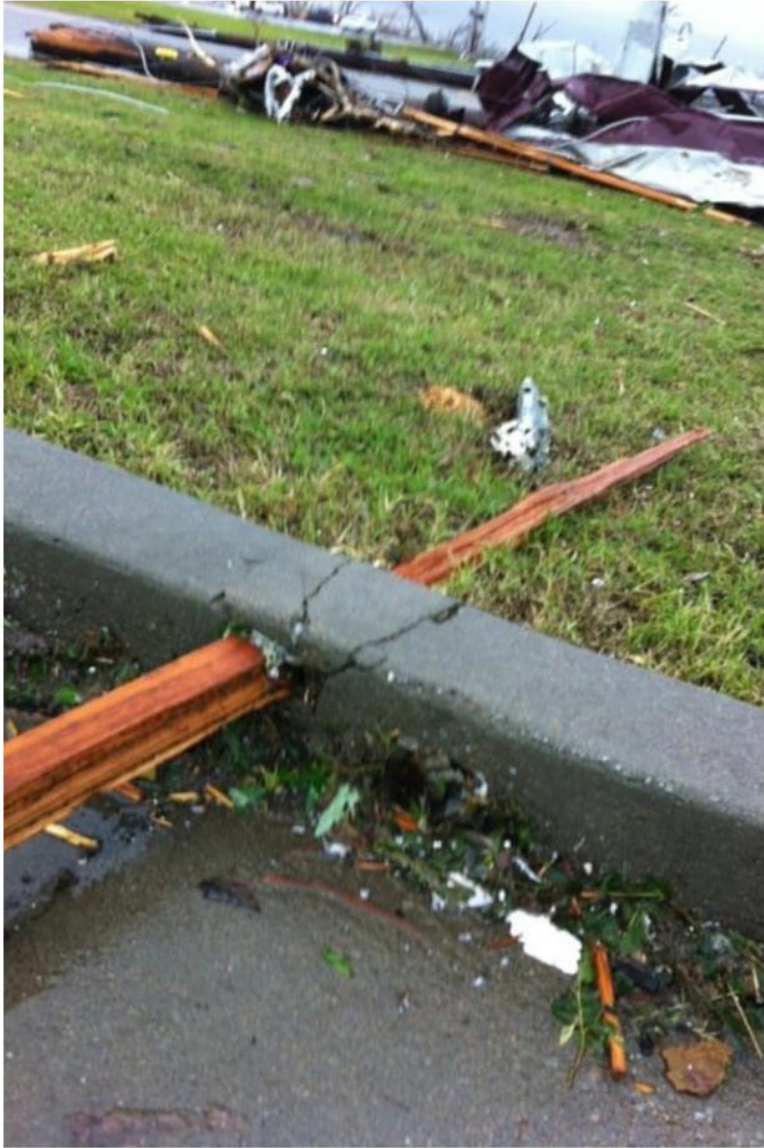
PHOTO 11: CEMENT CURB IMPAILED BY WOODEN BEAM
